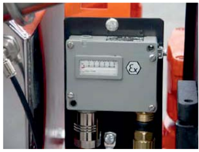
Ex Shut down pressure switch.
